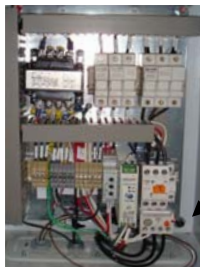
Control and power panel Fully wired and tested
